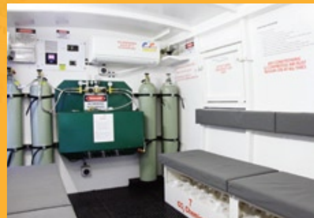
Interior of unit with Air Scrubber CO 2 removal
